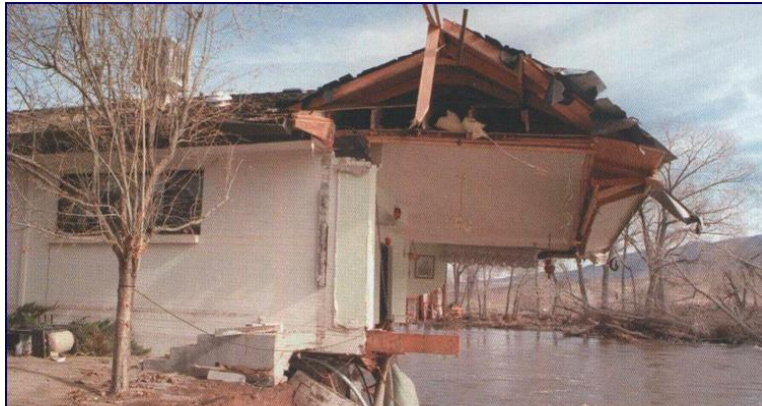
Impacts of Channel Migration on a House in Dayton during the 1997 Flood Event. (Photo courtesy of the Reno-Gazette Journal)
